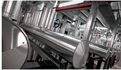
Cold water is pumped into horizontal rings of pipework serving cooling units
